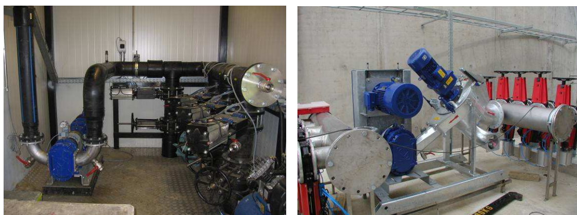
Figure 7.9 Pumping systems (AGRINZ 2008)
