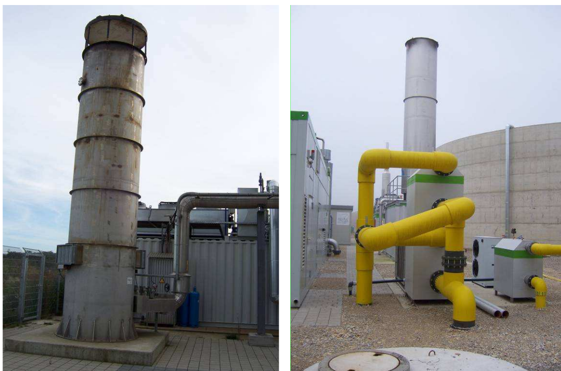
Figure 7.28 Modern biogas flares (RUTZ 2007)
